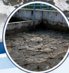
High Sludge Production
