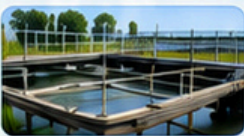
Aeration Tank ETP / CETP
